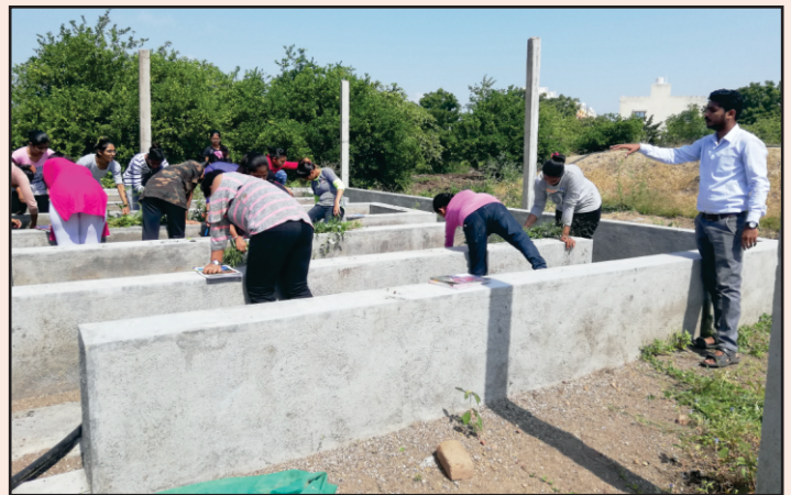
Community building the compost pits, where organic matter decomposes in the form of manure
